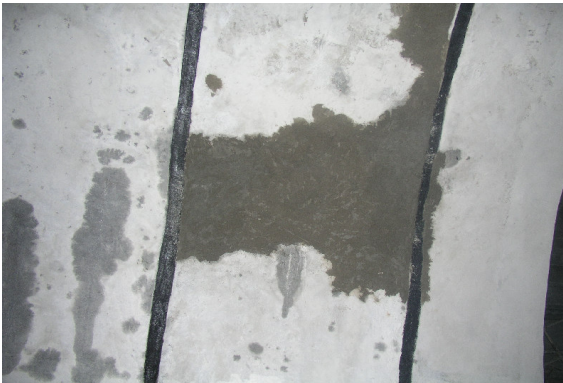
Figure 1. Active leaks at joint
